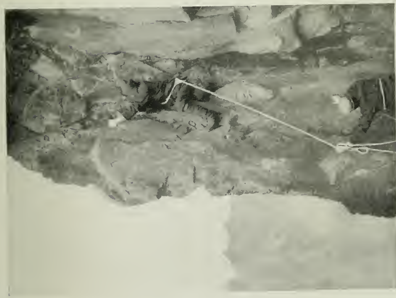
A STIFF CRACK. (Photo, G. P. Abraham.)
